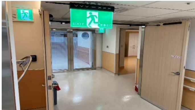
Emergency lighting and exit signs
