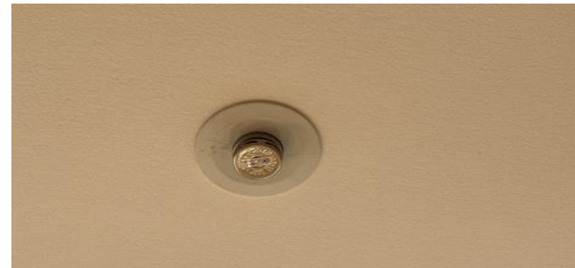
Automatic Fire Sprinkler System
