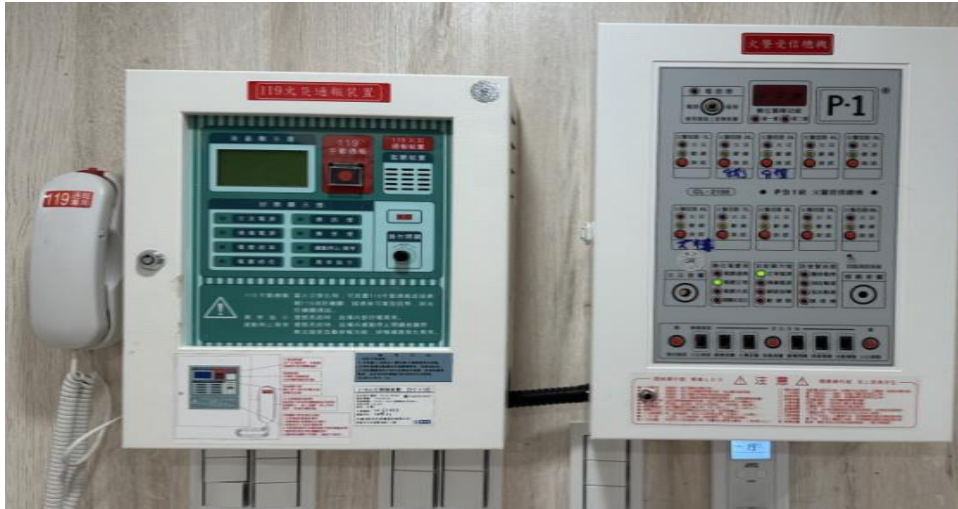
Fire alarm control panel and auto call to fire station
